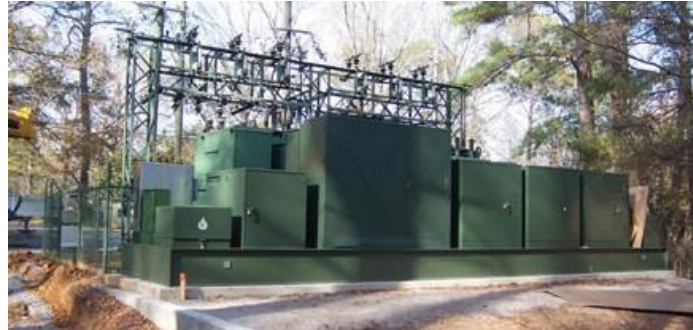
MITS installation in place of traditional overhead substation
