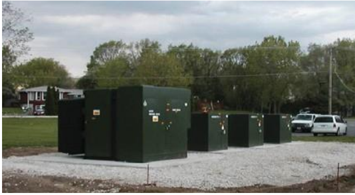
Utility substation placed in the middle of a suburb without the need for fencing and overhead lines
