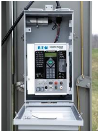
Door-mounted CL-7 single-phase control
